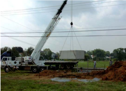
Septic Holding Tank
